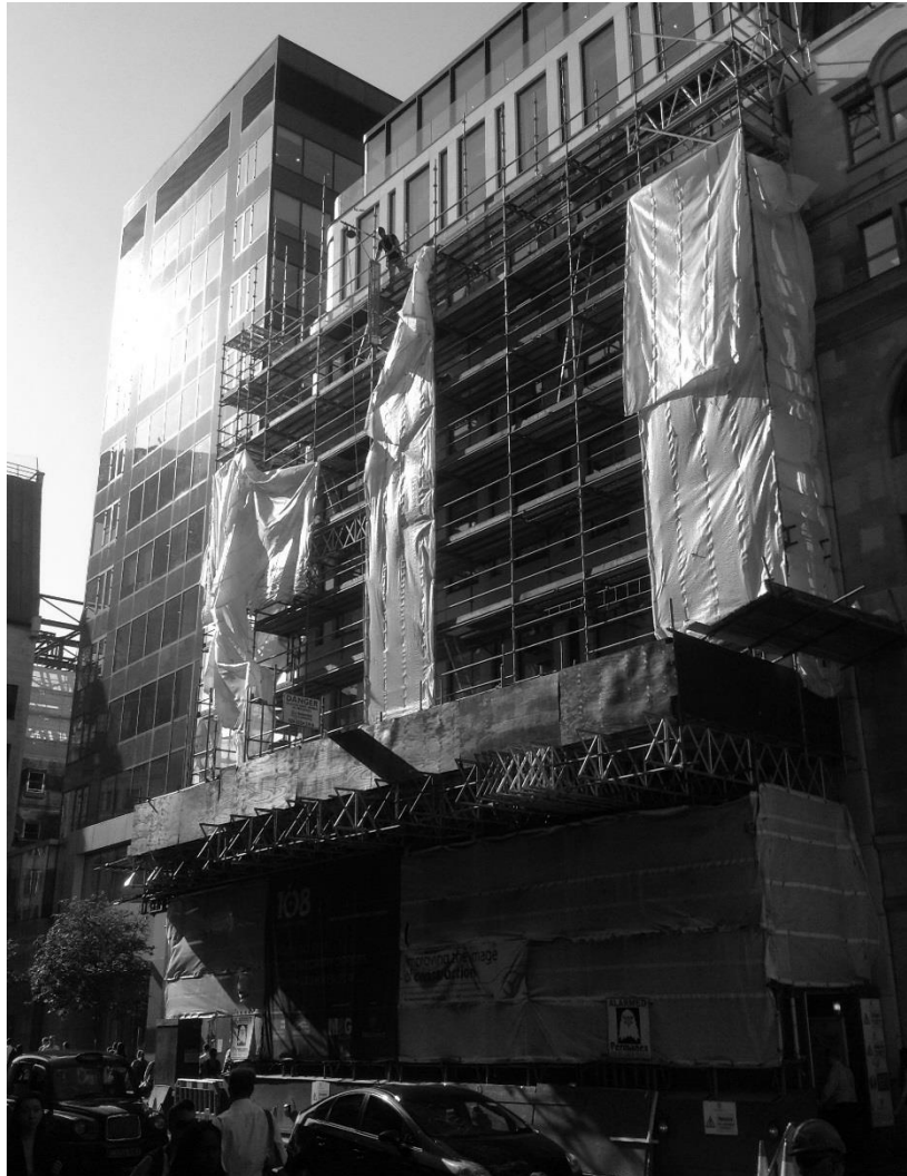
Photo 1: Risk of falling objects
